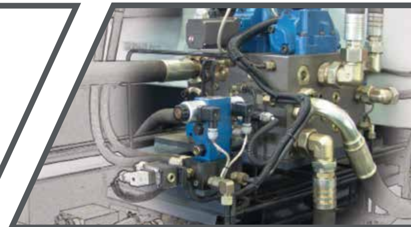
Hydraulic Valves Mounted Close to Actuators
